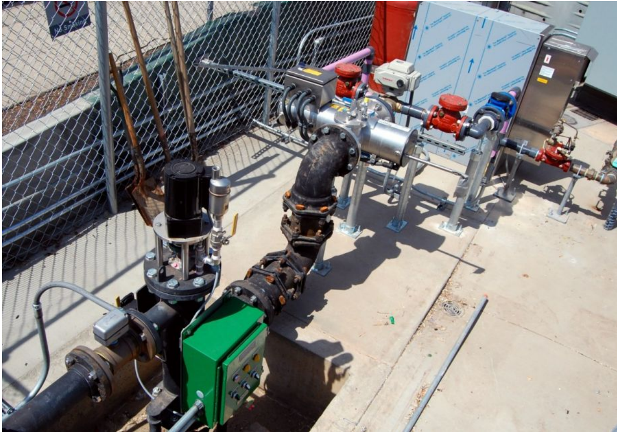
Treatment equipment at Los Amigos Park (Credit: City of Santa Monica)
